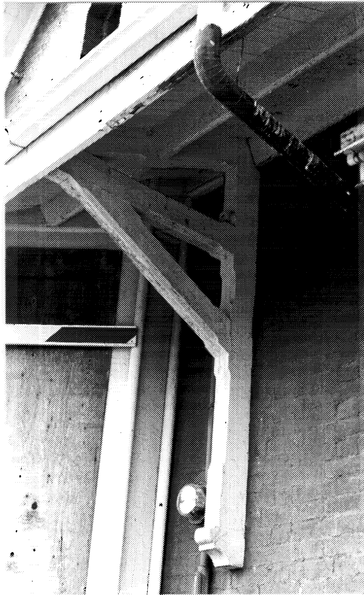
16 Detail of open timber support for narrow section of overhang, former CNR station, Ingersoll, as photographed in November 1992. ( Glenn J Lockwood, Ottawa. )
